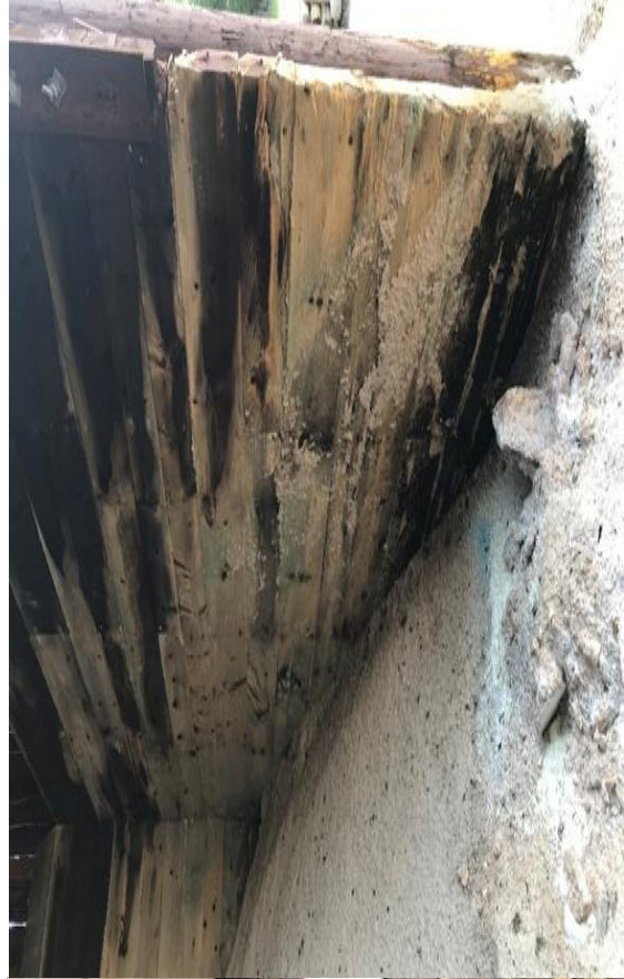
Belmont (314) – Deteriorated wall condition
