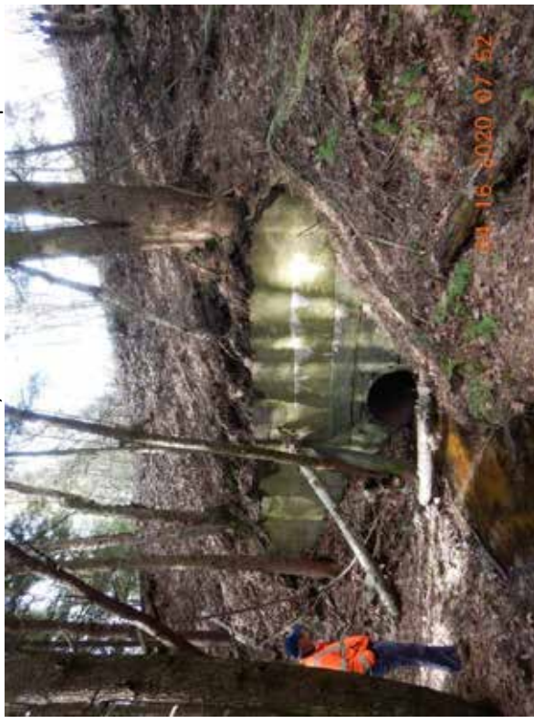
Concord-Lincoln Corridor, Canterbury Culvert MP C7.22 Vegetation Removal Required to Preserve Culvert Pipe Headwall Slope Retaining Structure
