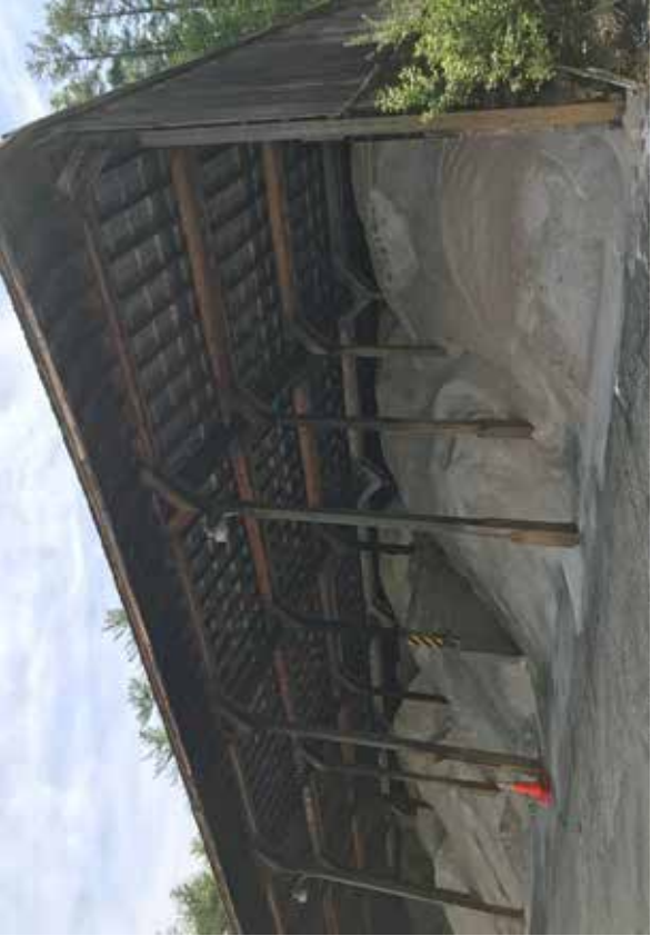
Warner (526) – Salt Shed inadequate capacity
