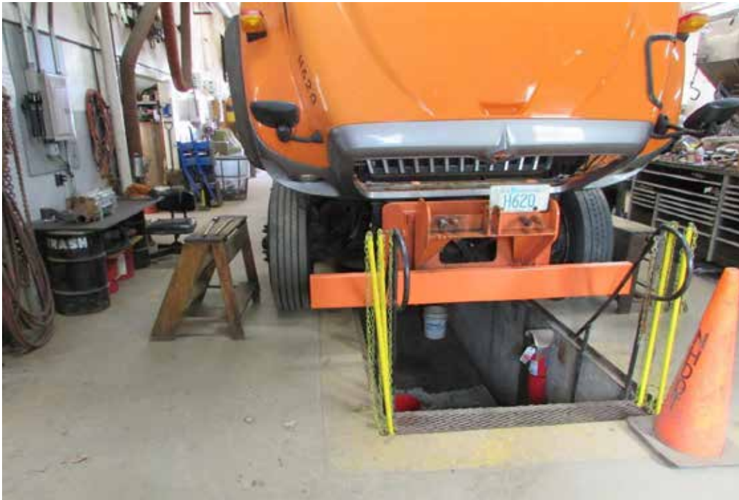
Lancaster – Low ceilings so employees work in a “pit”. The ceilings are too low to raise the dump body of have use for mobile lifts that would improve ergonomics.
