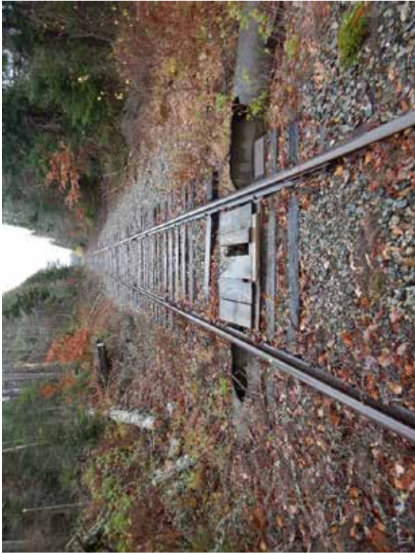
Mt. Division Railroad Corridor, Carroll MP 95.21 Culvert Pipe Failure
