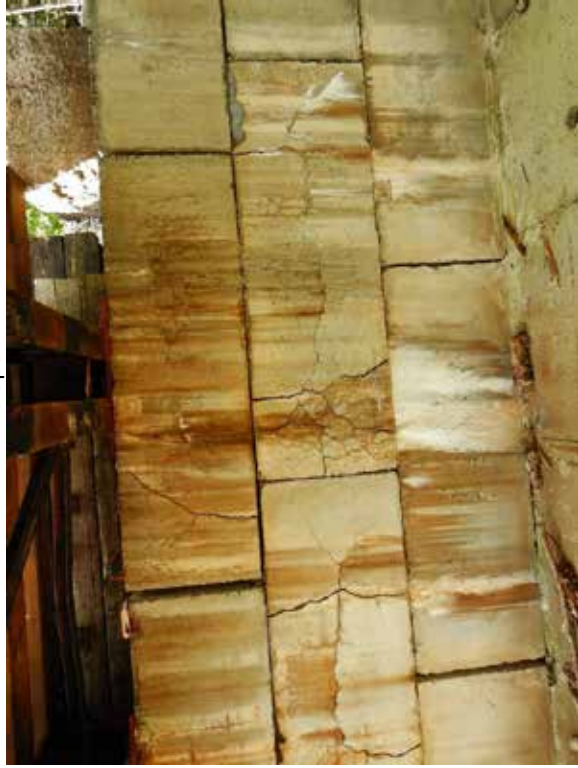
Mtn. Division Railroad Corridor, Harts Location Bridge #82.96 Failing East Abutment
