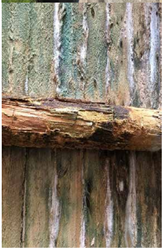
North Hampton (612) – Wall and post rot
