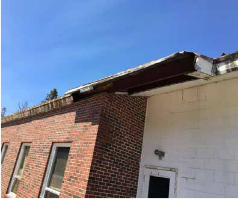
Close-up view of the holes in the trim and soffit where pigeons and animals gain access to the interior of the building.
